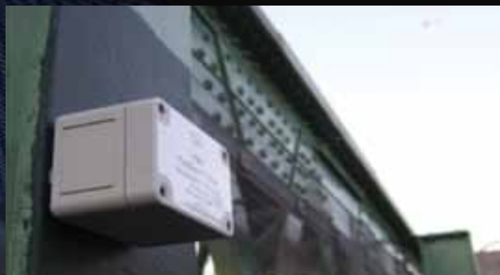
Senceive: Bridge monitoring (Network Rail)
