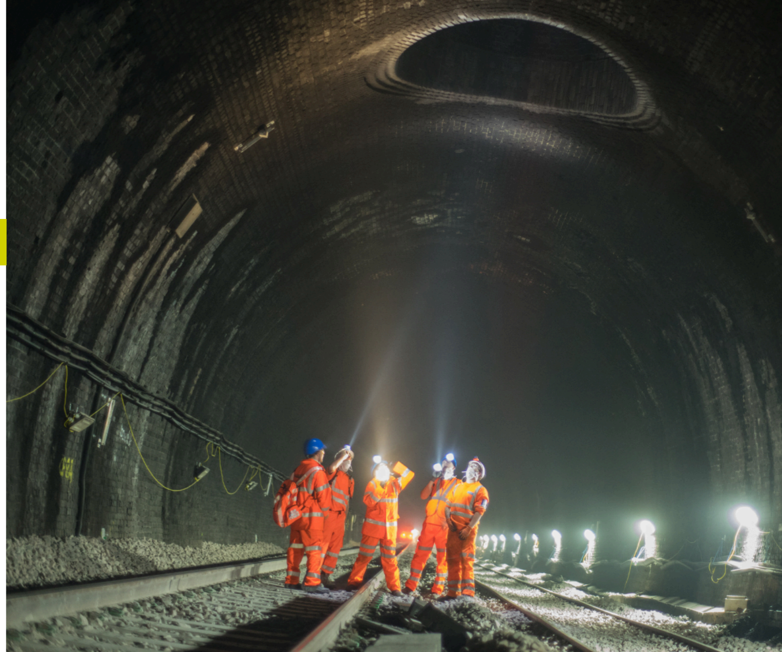
Senceive provides wireless solutions for railtracks, earthworks and structures.
